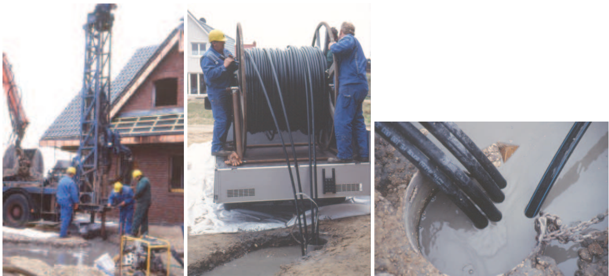
Fig. 6.14: Three steps of borehole heat exchanger installation: Drilling (upper left), inserting pipes (upper right), grouting (lower centre)
