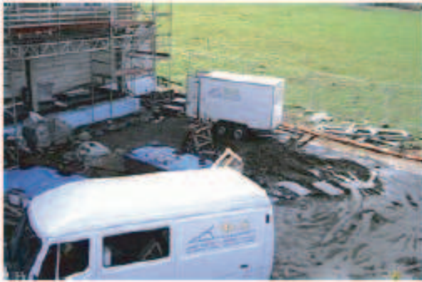
Fig. 6.23. Geothermal Response Test equipment on site (in trailer)
